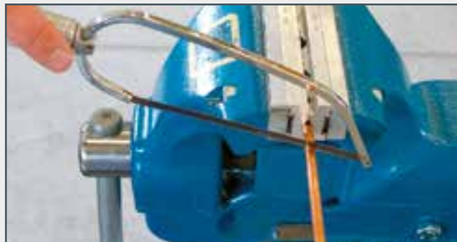
Determining the length of the pipe section. Here the additions for bends and flanges must be taken into account. Sawing off the pipe.
