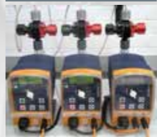
Precise addition of chemicals by use of industrial metering pumps
